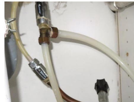
Messingfiting i rustfri installation
