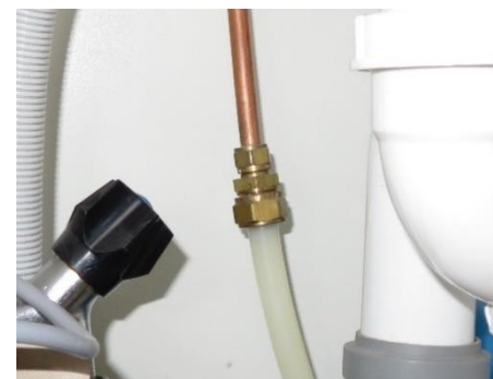
Messingfiting i rustfri installation
